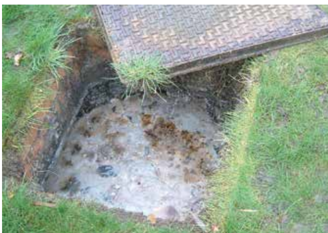
Fat building up in a manhole
