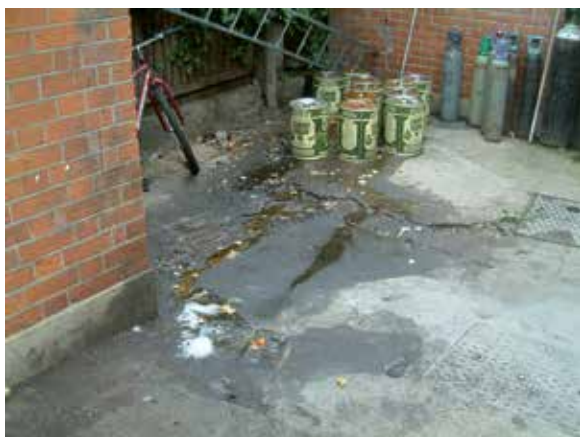
Avoid poor waste oil storage which could result in a sewer blockage or pollution incident
