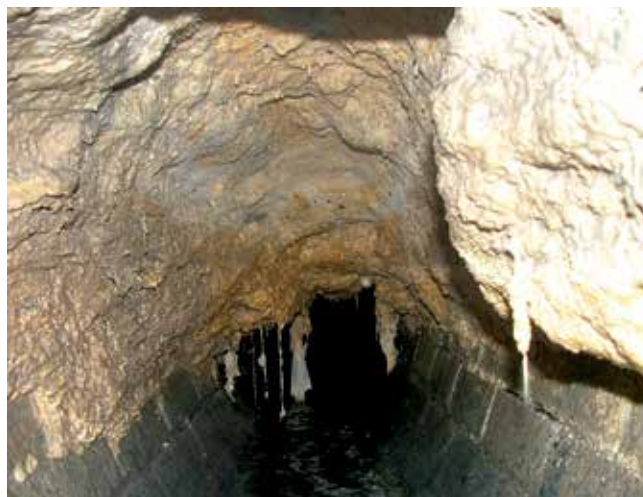
Fat beginning to block a sewer
